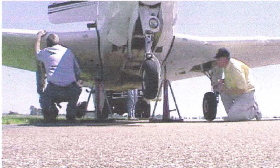
Notice that there is no tail stand. A couple of helpers simply balanced the tail in place for the few minutes it took to get the gear down and the jacks lowered.
